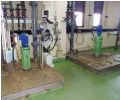
混和・凝集槽 Mixing & Coagulation Tank
