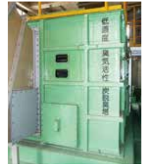
低濃度活性炭脱臭塔 Low Concentrated Deodorizing Tower
