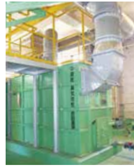
中濃度活性炭脱臭塔 Medium Concentrated Deodorizing Tower
